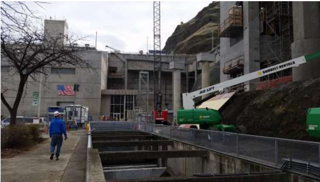
Photo 1. Installation of the above ground temporary potable water line and connection to the existing water line will occur on the north side of the ladder.
